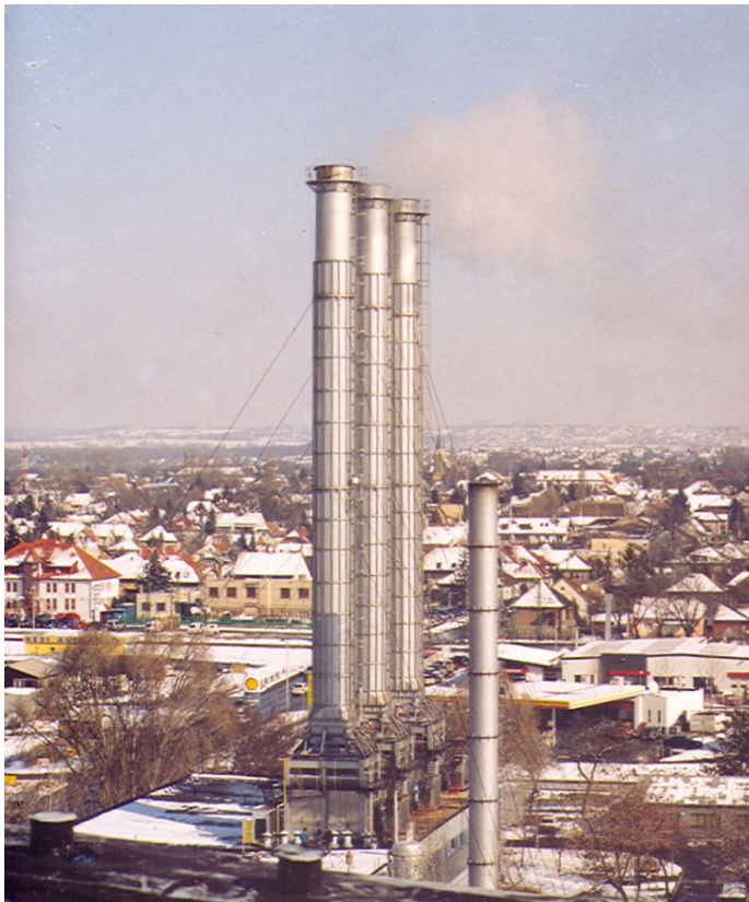
Photo 1. The testing object: 150 MW heating plant in the 14th district of Budapest
