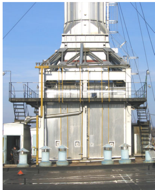
Photo 3. Boiler, confusor and lowest part of the stack.
